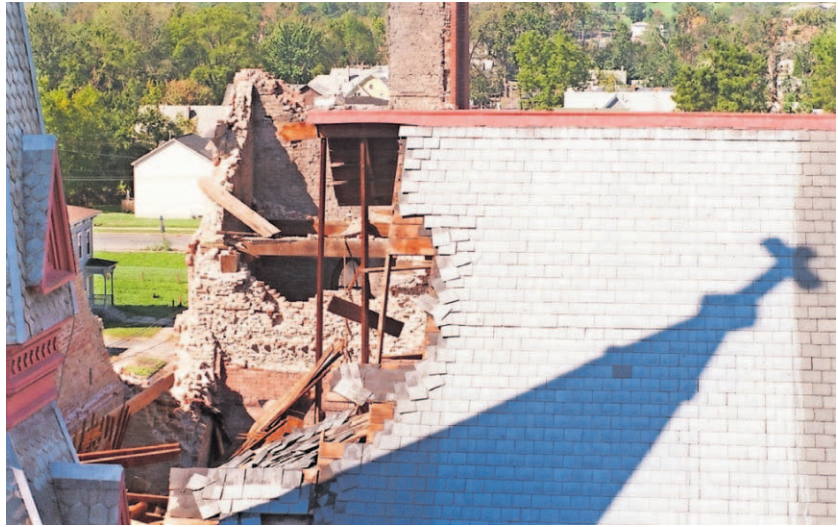
The Labor Day storm of 1998 caused widespread damage, including this hole in the roof of St. Lucy's Church on Gifford Street on Syracuse's Near West Side. Post-Standard file photo
