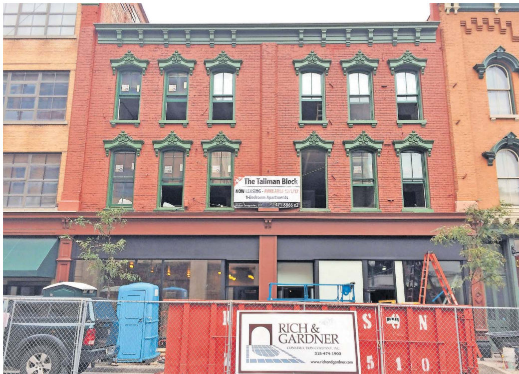
The Tallman Block building, seen here from West Fayette Street in Armory Square, had a fourth floor that was demolished in the 1930s. The building's upper two floors are being turned into apartments. Rick Moriarty, rmoriarty@syracuse.com
