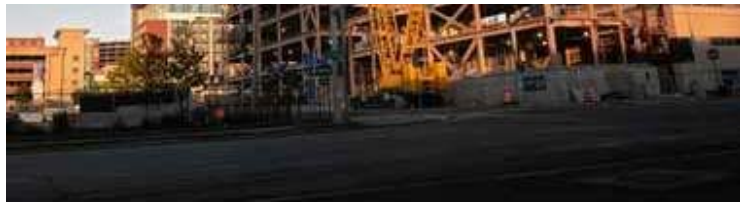
A $100 million cancer center is under construction as part of Upstate Medical University in the shadow of Interstate 81.
