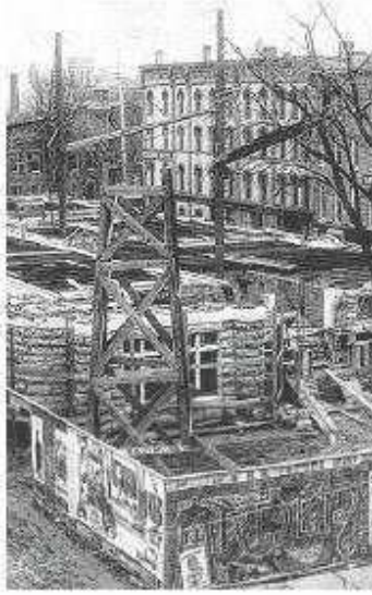
City Hall under construction in 1889. Placing steel for the second floor. (OHA)
