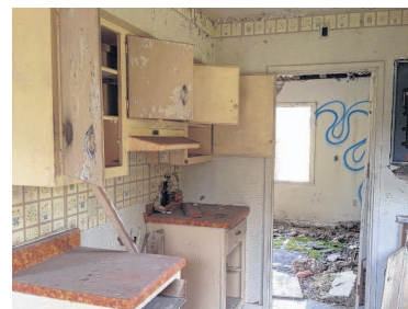
Time has not been kind to the complex that once housed military families at Hancock Air Force Base in Cicero. Demolition of the long-abandoned housing was recently completed. (Rick Moriarty / rmoriarty@syracuse.com)
