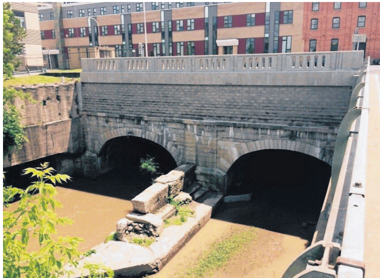
This view of the historic bridge that carried the Erie Canal over Onondaga Creek is off limits to the public because of safety concerns. A new park on top of the bridge will offer a view of the creek, but not the stone arches. (Sean Kirst / skirst@syracuse.com)
