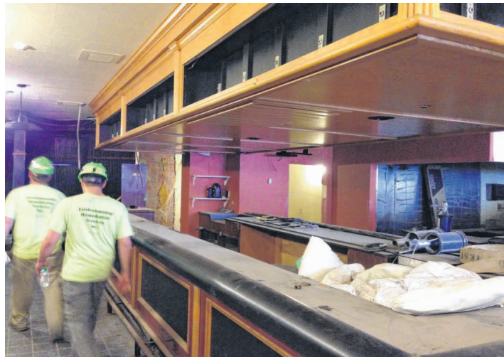
Construction workers walk past the bar in the former Rainbow Lounge in the Hotel Syracuse. The art deco circular bar, a notable feature of the lounge when it opened in 1937, was replaced in the 1970s. (Rick Moriarty / rmoriarty@syracuse.com)
