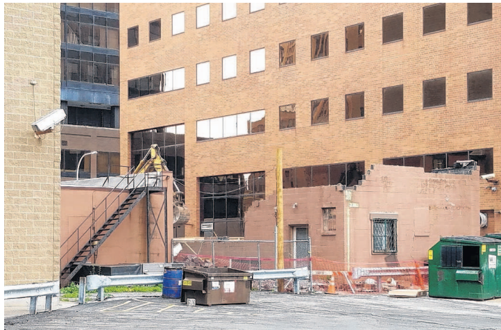
The building at 318 E. Fayette St. in Syracuse was being demolished on May 22. It was built as a home sometime before 1851 and was one of the city's oldest buildings. (Pamela Priest / Onondaga Historical Association)
